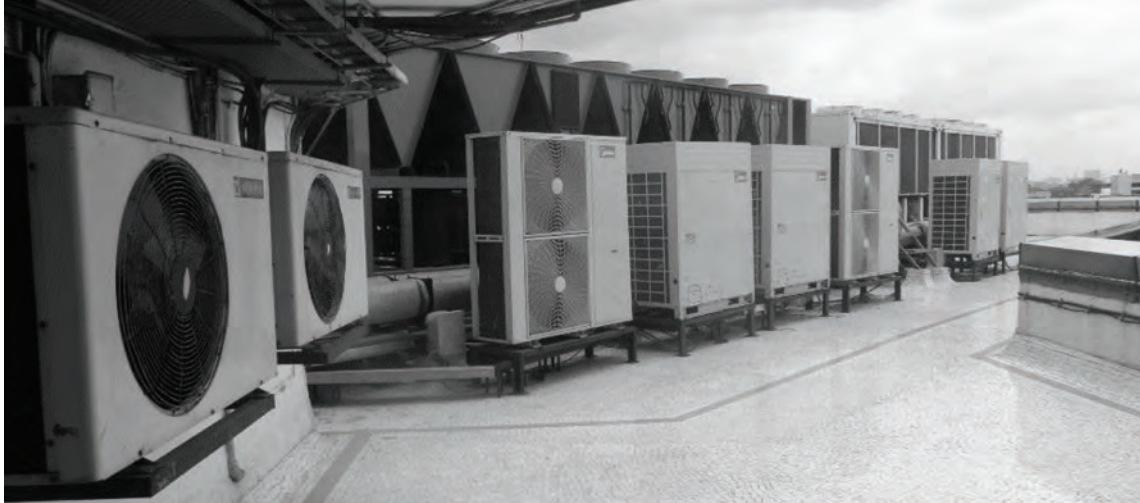
Energy efficient chillers installed in a certified green project.
