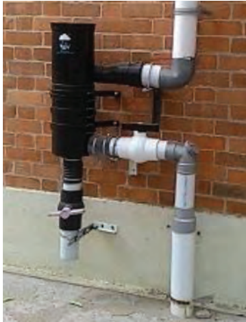
Rainwater down pipe with filter & first flush valve
