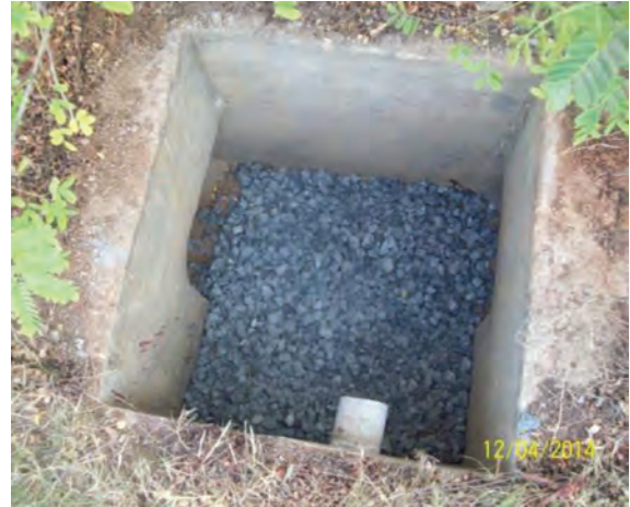
Rainwater collection chamber with filtration media
