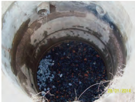
Rainwater recharge pit
