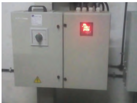
A dedicated sub-meter installed for a fit-out to measure its space conditioning energy use at Platina Tech Park, Chennai
